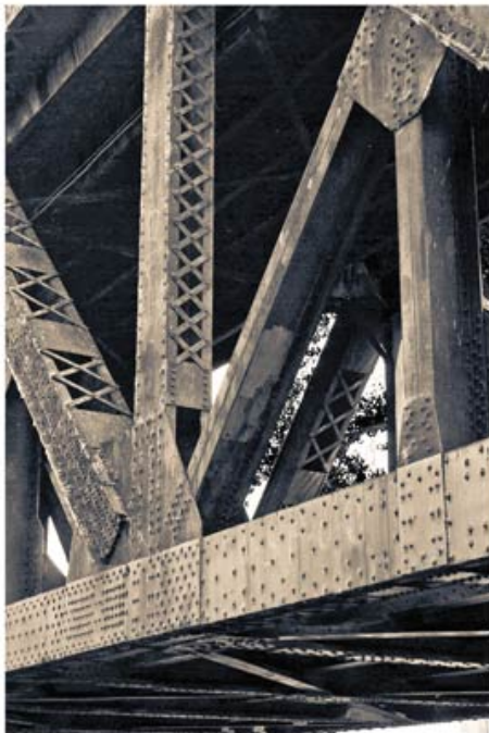
Rusty Trussle - TR18081
