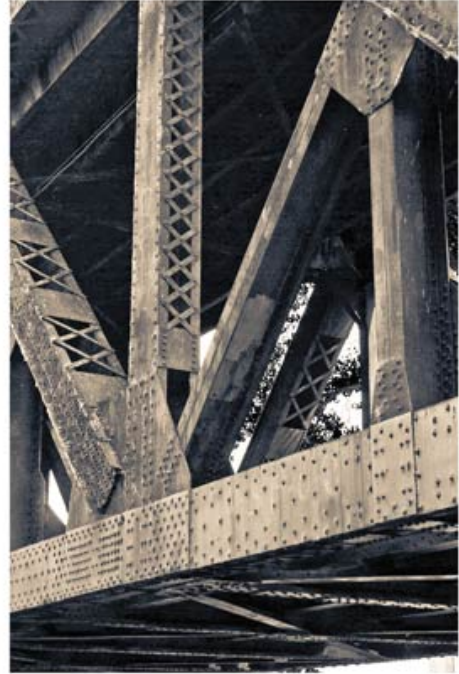
Rusty Trussle - TR18081
